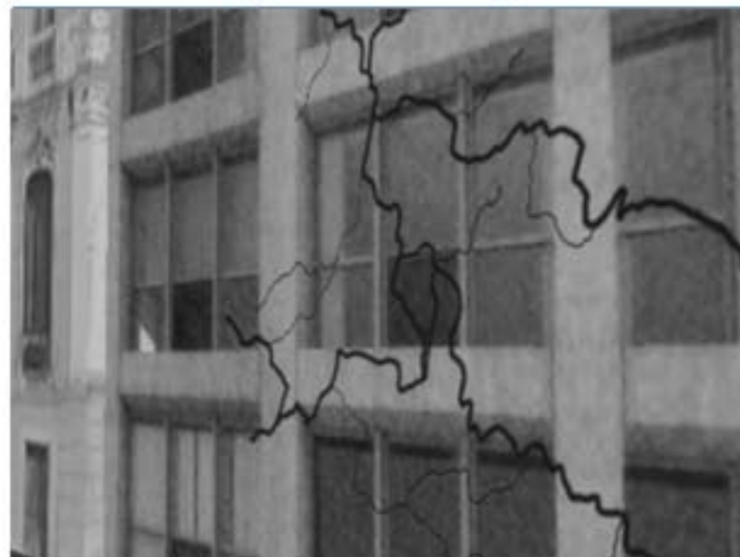
Cracks run up the sides of the buildings.
